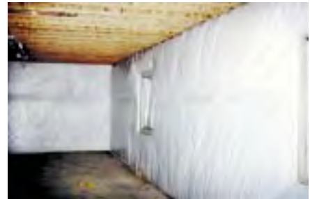
Photograph 3 Blanket insulation with impermeable vinyl interior surface
