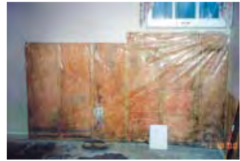
Photograph 5 Frame wall with interior vapor barrier resulting in mold, decay and odors
