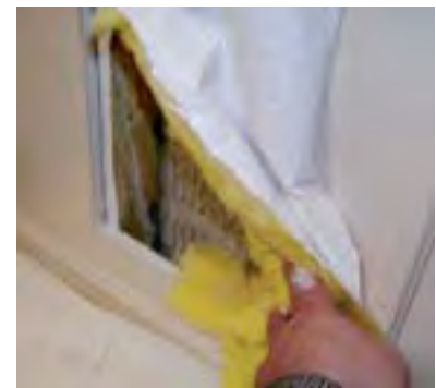
Photograph 7 Mold with blanket insulation
