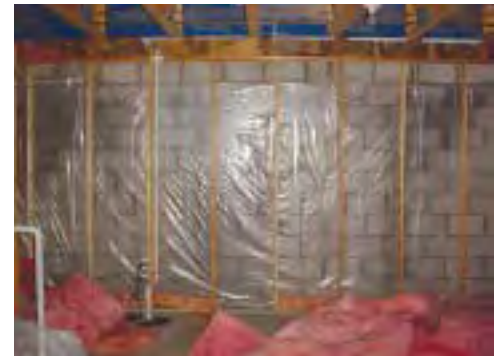
Photograph 6 Water trapped behind polyethylene installed directly against foundation wall
