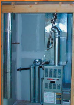
HVAC equipment located within the building envelope.
