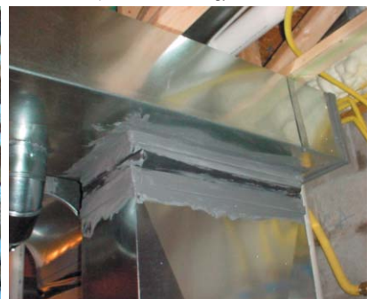
Sealing ductwork with UL-181 approved mastic, as shown in the photo below, is one component of an hvac optimization strategy.
