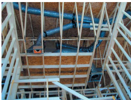
A typical home with two HVAC systems can have a web of ducts running from the system in the attic, as shown in the photo below.
