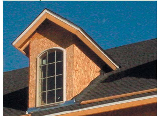
The intersection between the roof and the wall of this dormer should have a good water management strategy.
