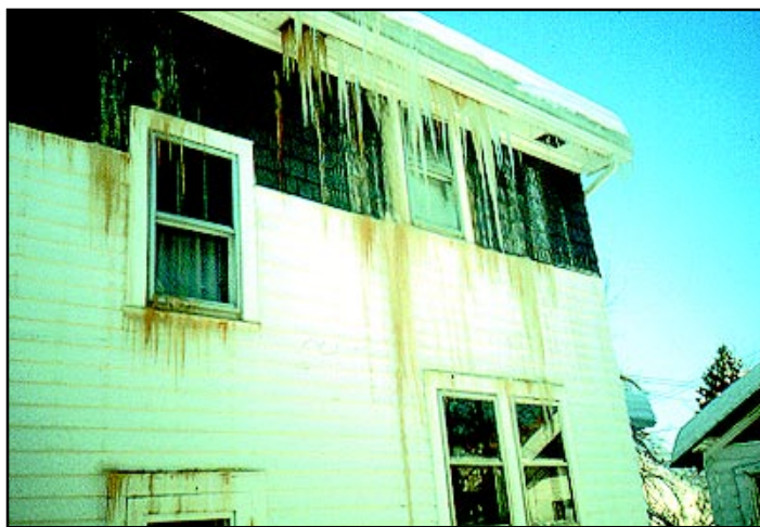
Heat loss into attics from air leaks, ducts or flues can lead to ice dams, even when the attic is vented.
